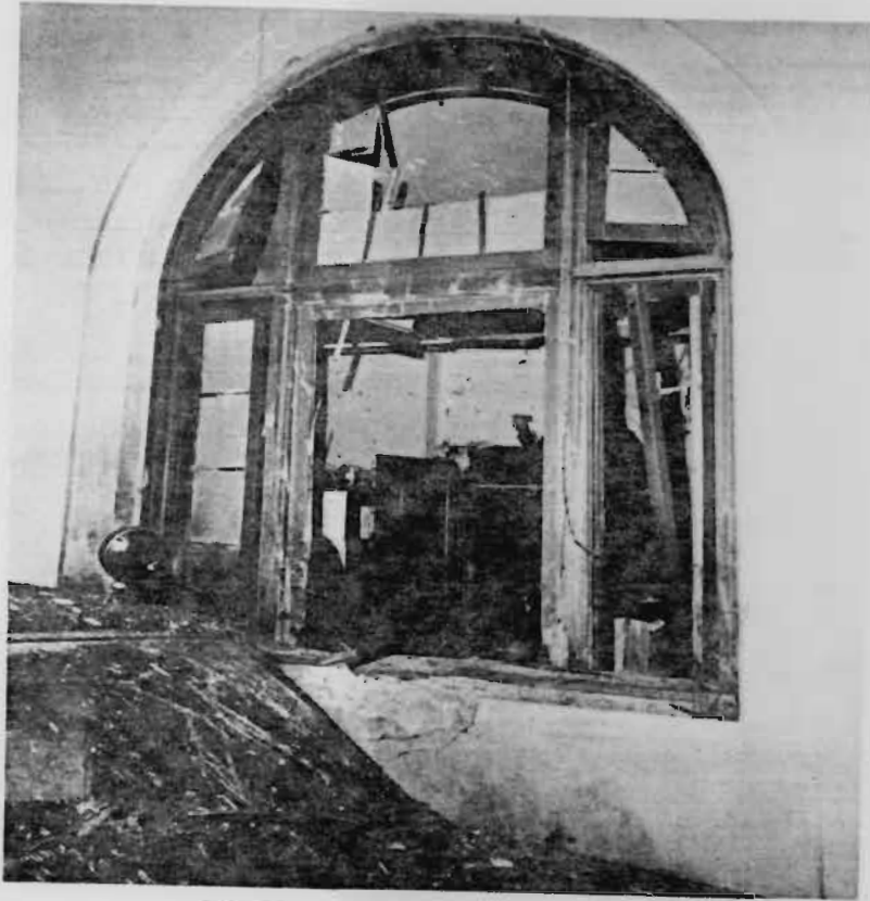
Bombed police station, San Francisco.
