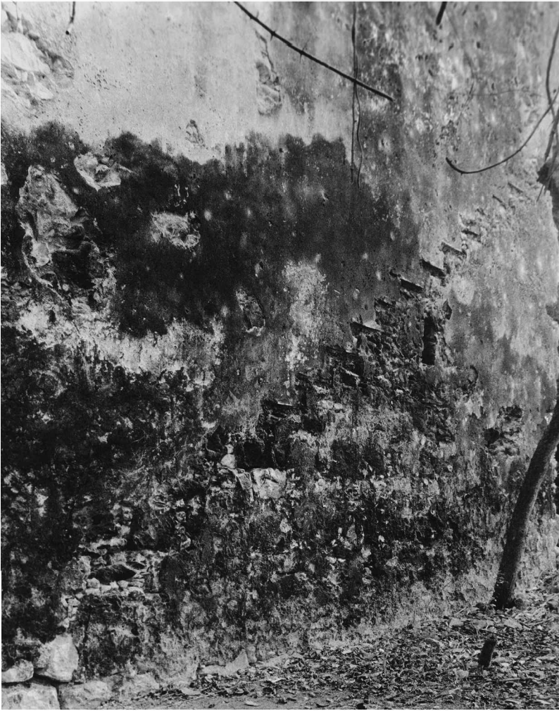
Plate 2 Traces of a stairway on the southern exterior wall of slaveholder's house.
